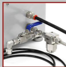
Compressed air and CO2 supply connections
